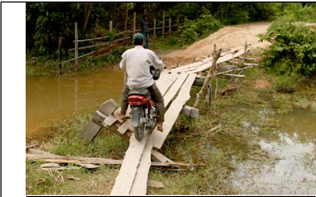
Replacing this dangerous old bridge.....
